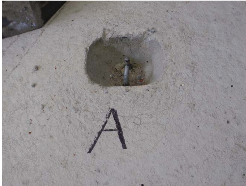
Figure 4 – Sample A Failure
