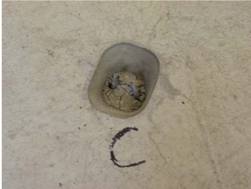
Figure 6 – Sample C Failure
